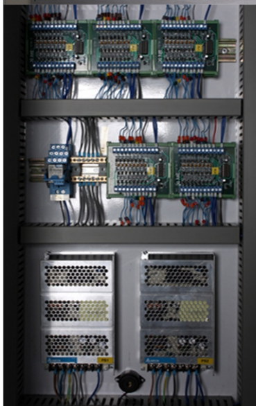
View Of Wiring RHS Panel
