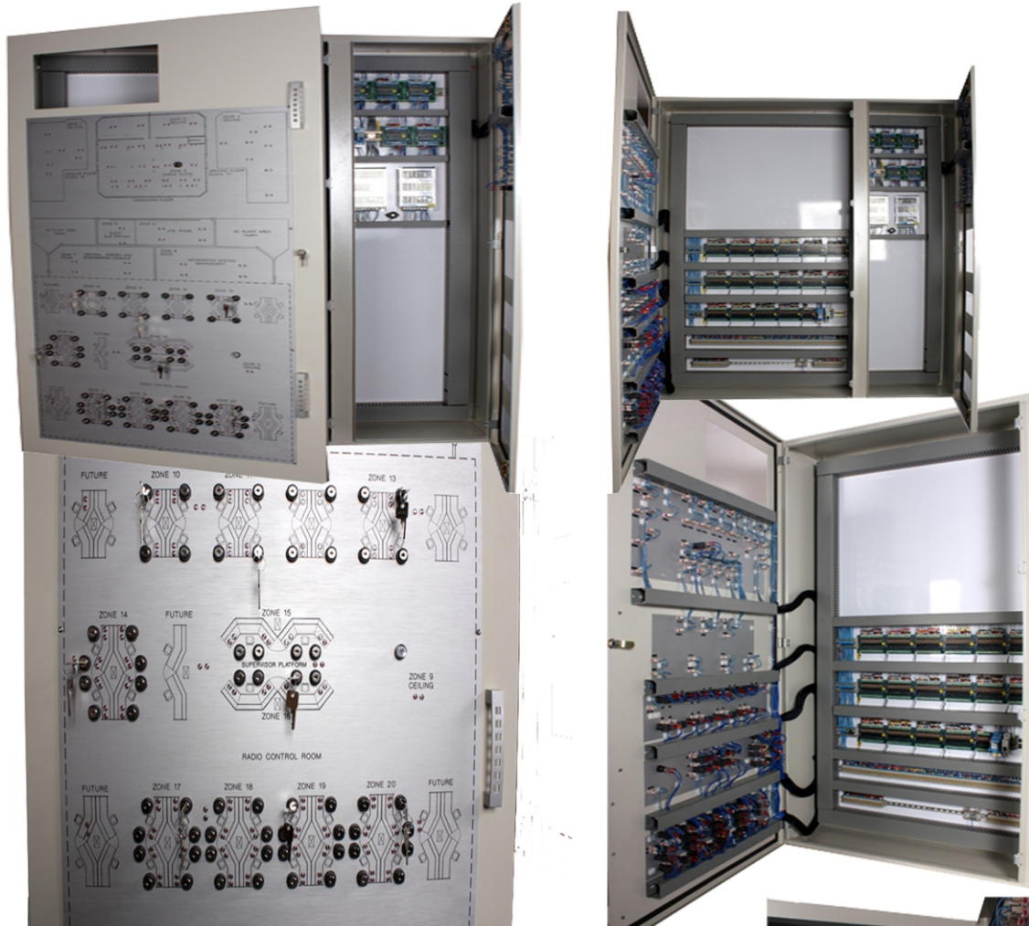
Custom Turnkey Mimic Panel
